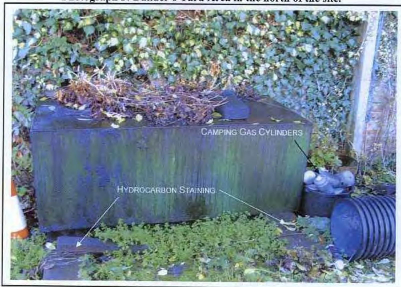
Photograph 4: Waste Oil Above Ground Storage Tank.
