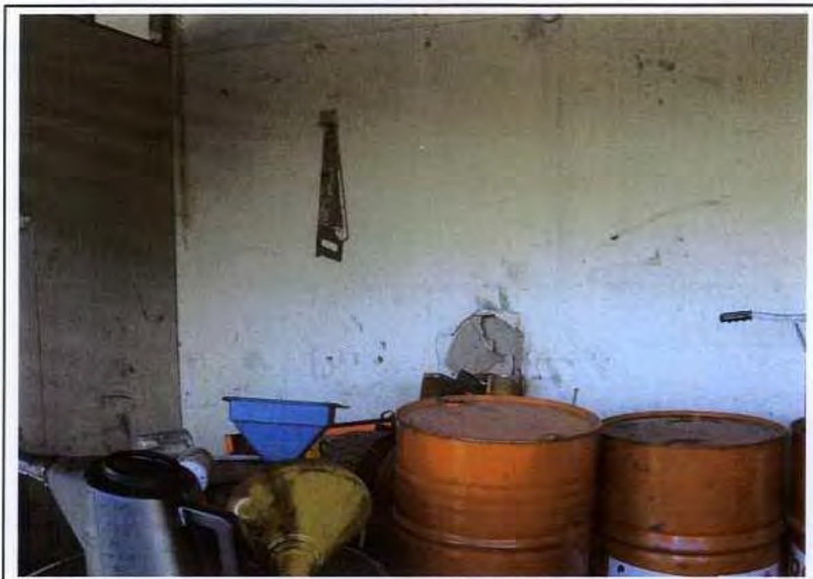
Photograph 7: Taped damaged areas in pACMs Insulation Board within the open fronted workshop building.
