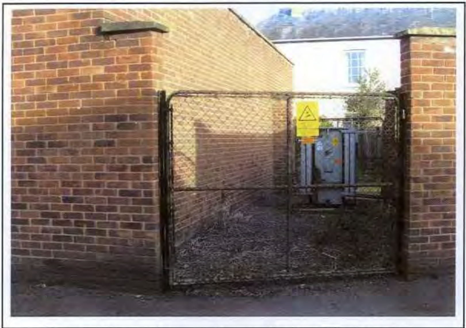
Photograph 5: Transformer to the east of the Electricity Substation.
