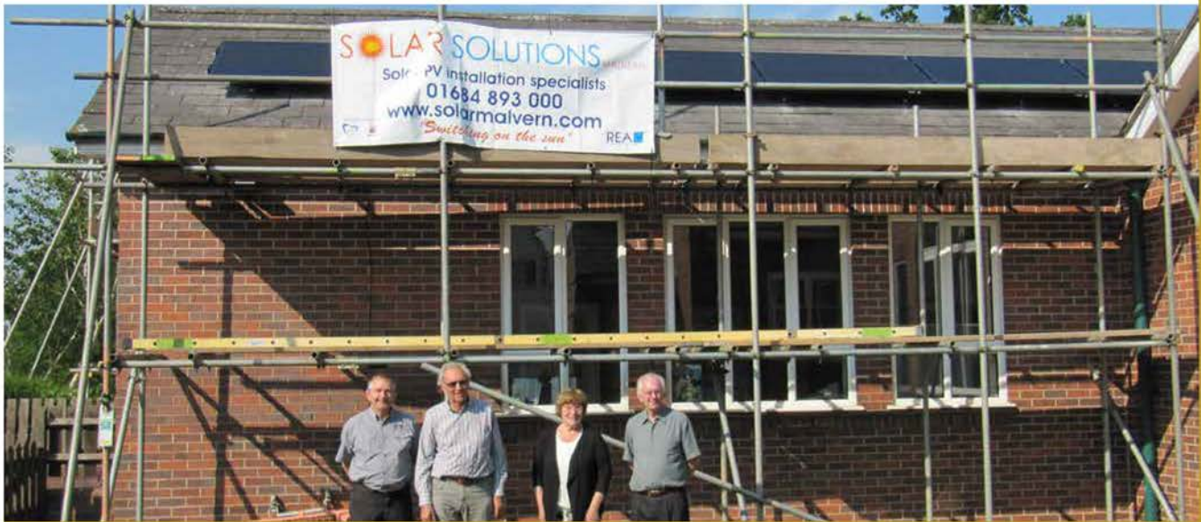
Colwall village hall Solar Panels
