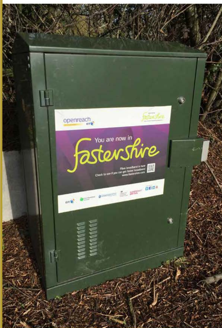
Telecomms cabinet, Near Ledbury
