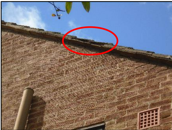
Plate 3: Showing missing verge mortar on the eastern gable of the house.
