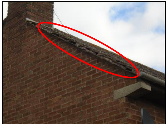
Plate 4: Showing missing verge mortar on the western gable of the house.
