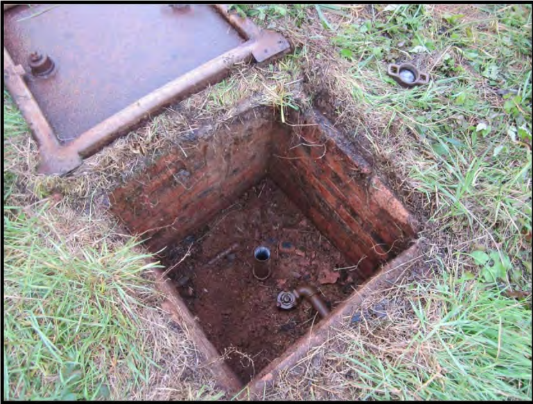
Photograph P3 : showing UST fill-chamber
